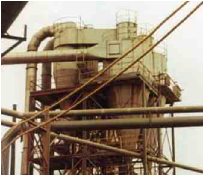
Wear resistant Quad Cyclone in incineration plant
