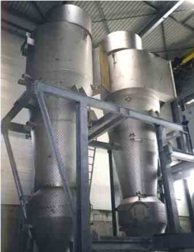
Heated Twin Cyclone for slurry dedusting (74.000 m 3 /h)
