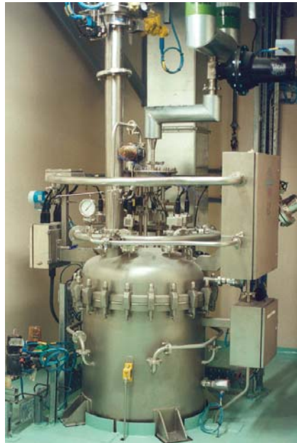
Typical custom built CIP filter
